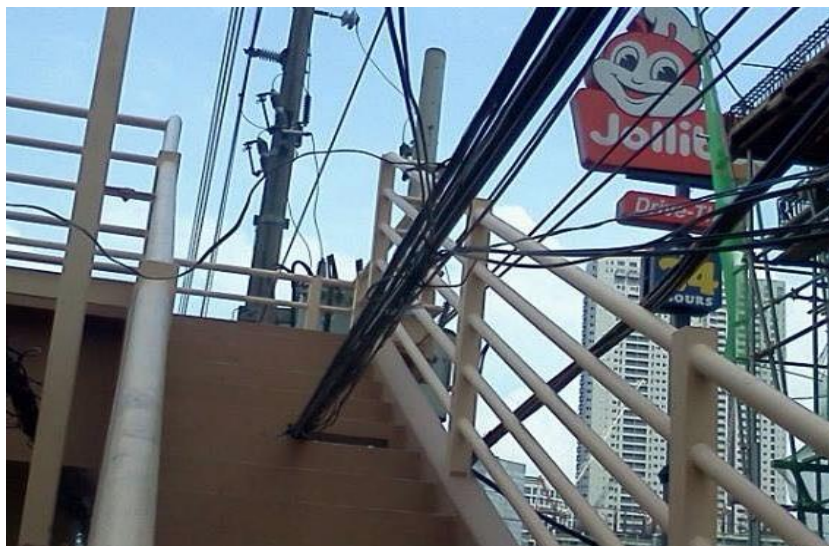
Figure 2. Footbridge with electrical wires through it in Libis, Quezon City (© Takayama)
