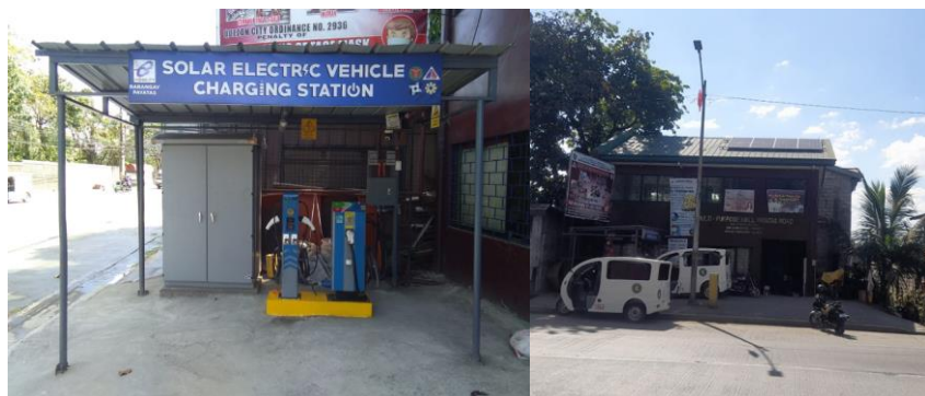
Figure 8: Actual pictures of solar e-trike fast charging station at the Environmental Office Building
